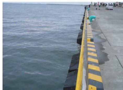
The N Wharf in the same area designed according to the revised specifications is in good condition after the 2011 East Japan earthquake
