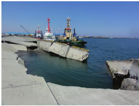
Damage and erosion of sheet pile wharf (No.1 quay of Xiangma port)
