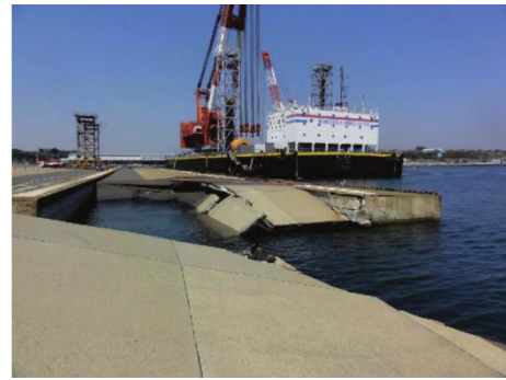
Collapse of the corner of gravity wharf (- 10m) (the 4th quay of Hitachi port, Ibaraki port)
